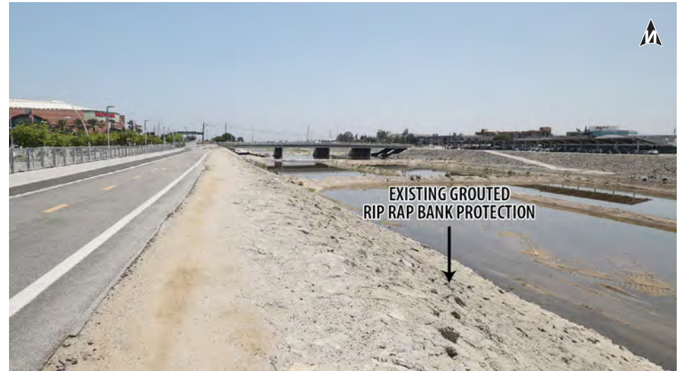
▲ From west bank of river, south of Katella Ave. Photo showcases what the existing 2:1 grouted riprap slope looks like throughout the majority of the corridor.
