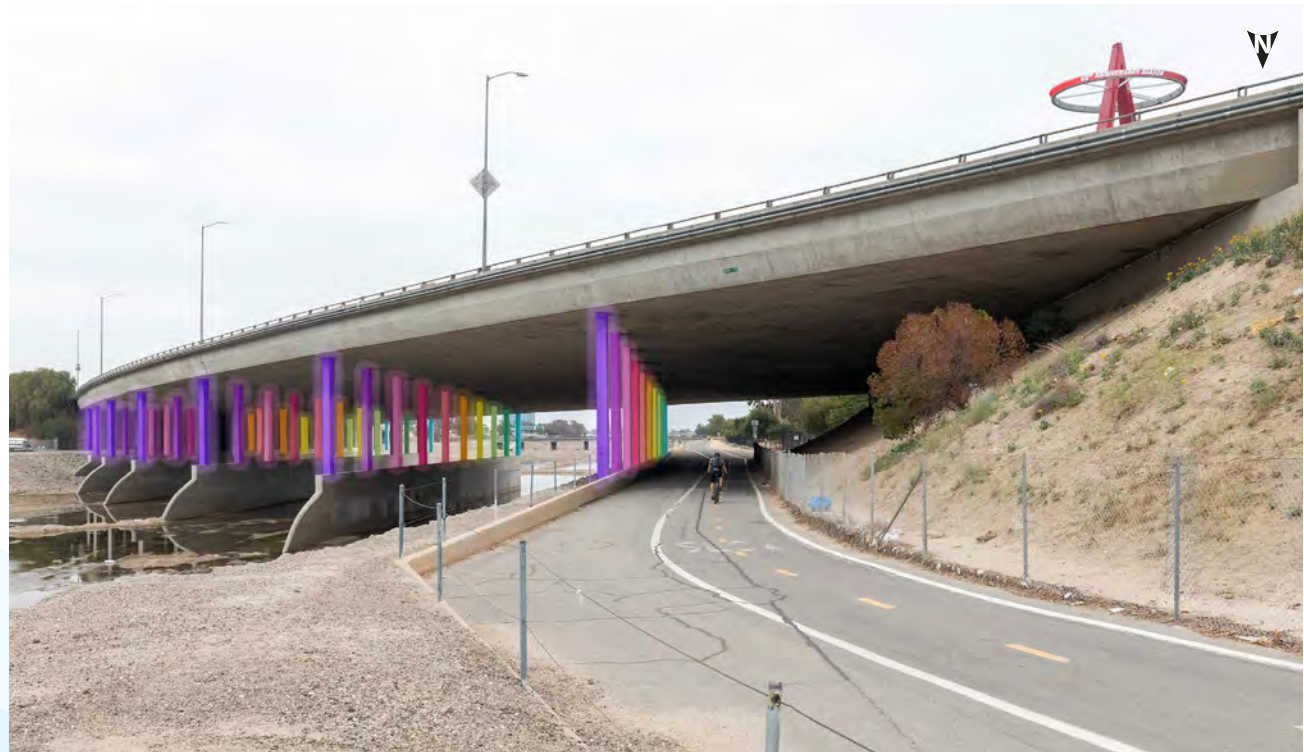
TOP: From west bank of SART, north of Orangewood Ave. bridge. 15A Sample rendering of art placed on bridge pier columns featuring indigenous fish species.
