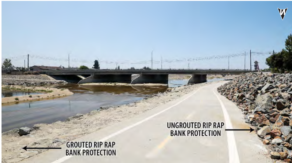
▲ From west bank of river, north of Katella Ave. bridge (view of undercrossing ramp). Photo shows areas of grouted riprap versus loose riprap above the riverbank.
