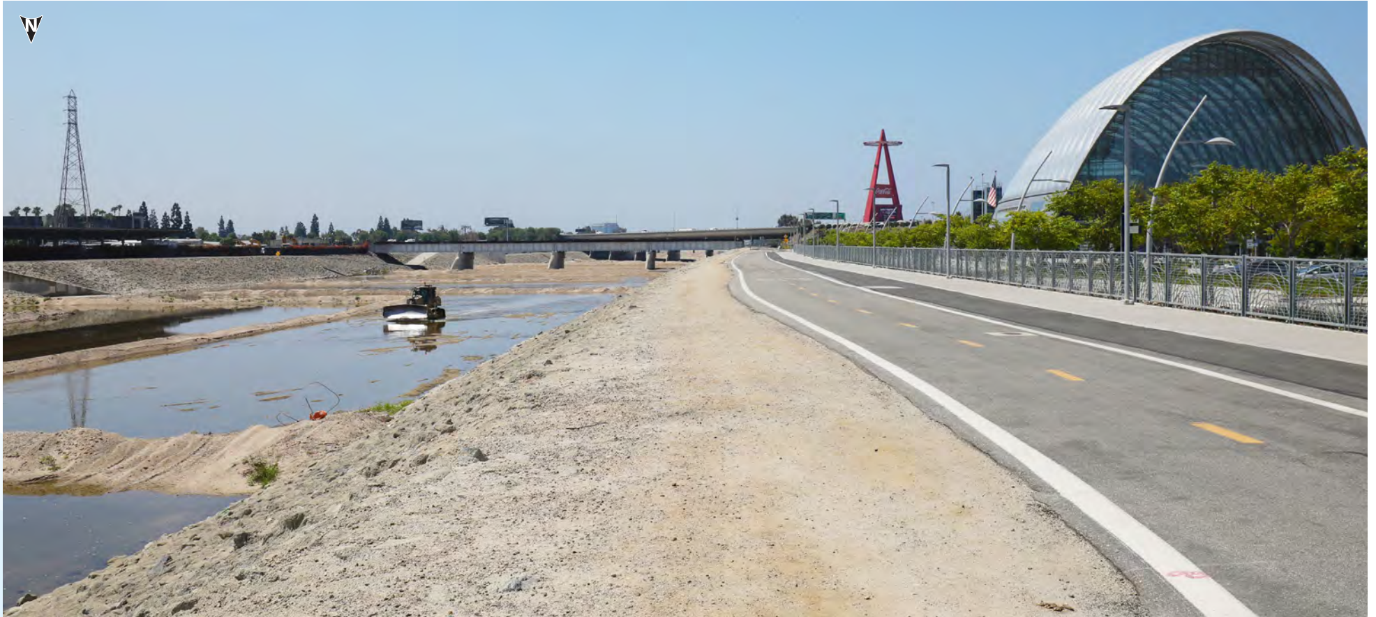
▲ From west bank of river, south of Katella Ave. near ARTIC parking lot. Impoundment structure eliminates need for OCWD to continually grade "T" & "L" levees in the bed of the Santa Ana River.
