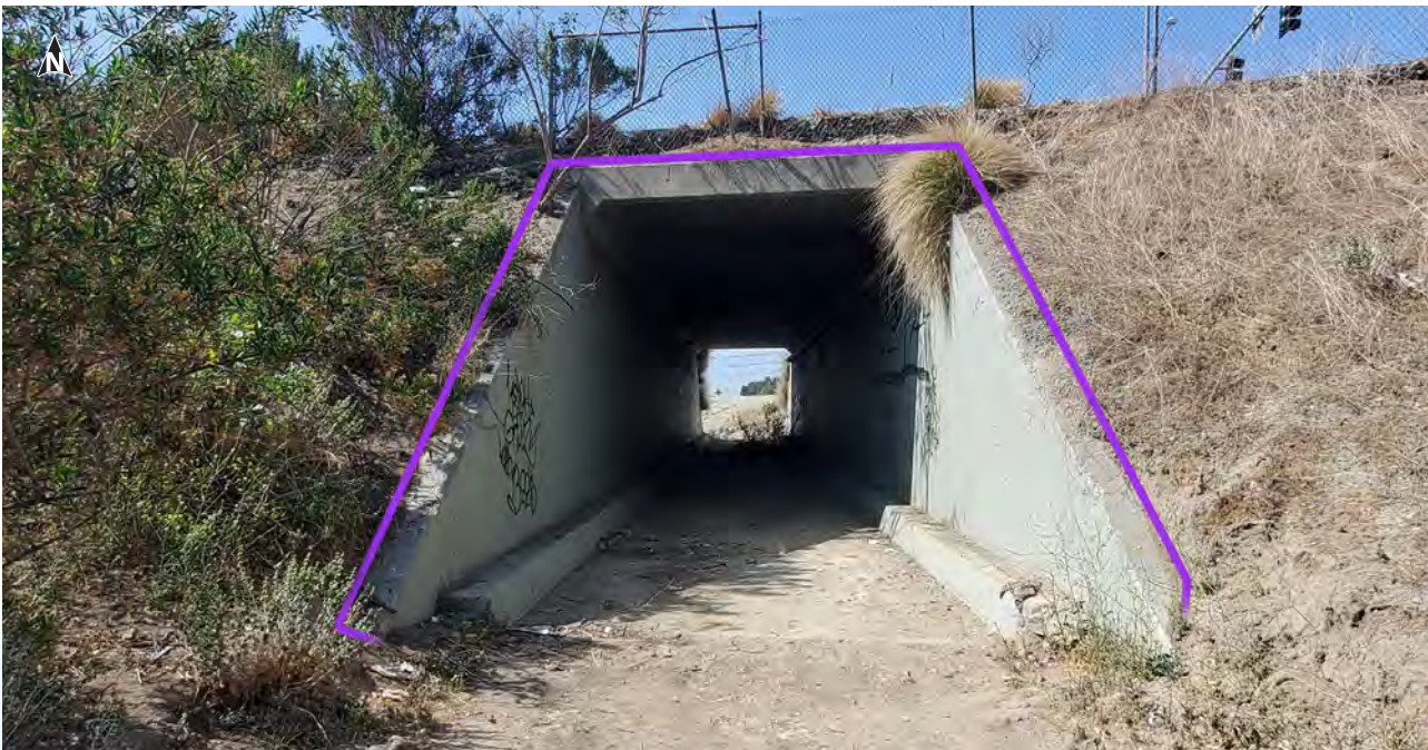
▼ View from south side of Ball Rd., east of Phoenix Club Dr. – Existing 14' x 14' RCB culvert repurposed for grade separated undercrossing.
